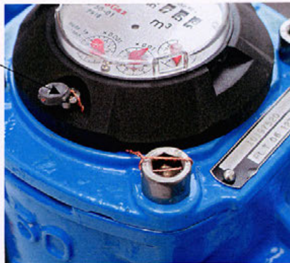
Picture No.2 Emplacement of the seal for security measures
