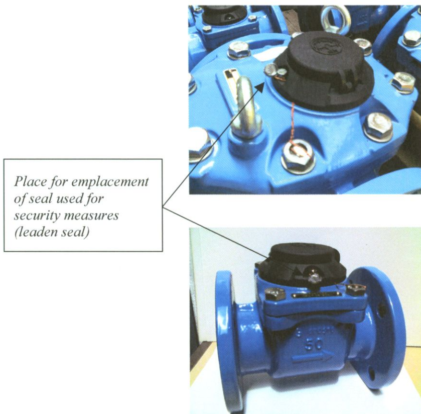
Picture No.2 Emplacement of the seal for security measures
